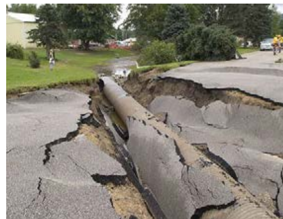
Damage to a road caused by flood water. Photo courtesy of Wikimedia Commons.
