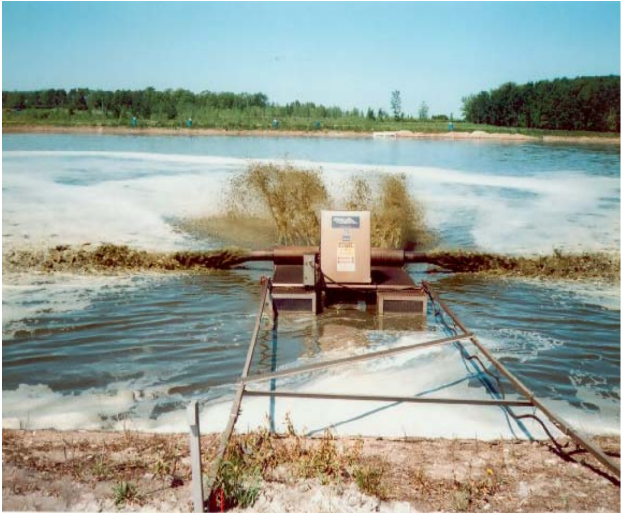
Figure 3. Excel Dairy Aerator.
