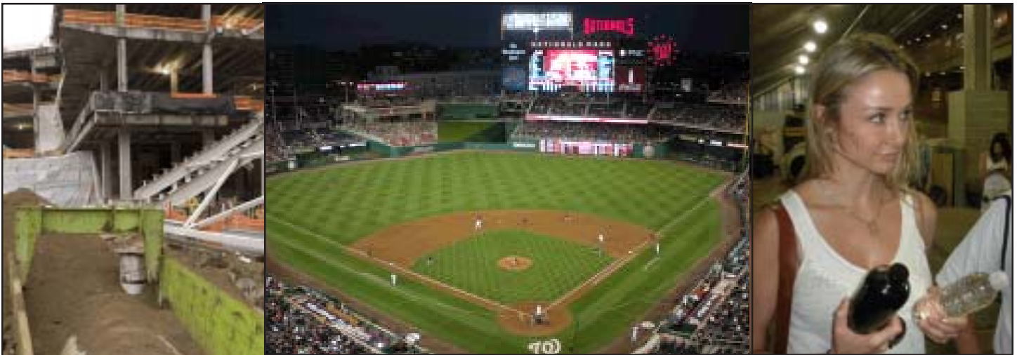
Left: Installation of the culverts under the warning track at Target Field in November 2008. Middle: Nationals Park in Washington, which was the greenest ballpark in the country until it was surpassed by Target Field. Right: Alexandra Cousteau and her international Blue Planet team toured Target Field and its water treatment system on July 3, 2010, as part of a 100-day, 1,450-mile expedition. The bottle in Cousteau's right hand contains water from the wet well; the bottle in her left hand contains water that has passed through the filtration system.
