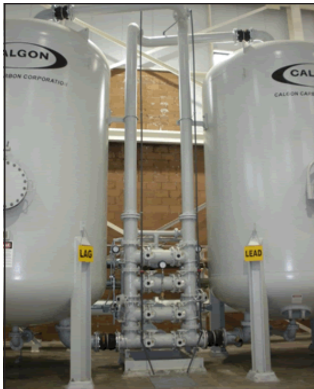
The filters use a lead-lag system.
