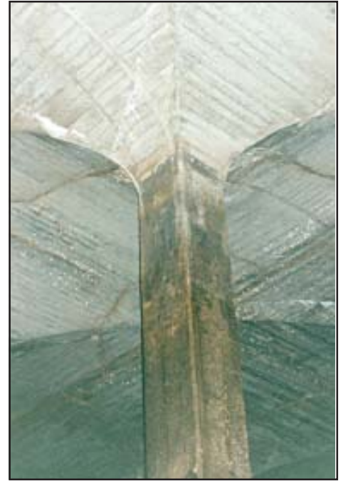
The roof is of the groined arch type supported by 21 inch square columns.
