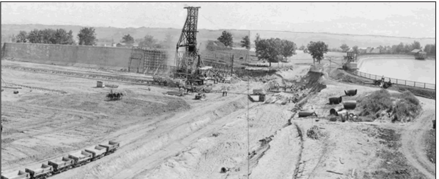
Photo from 1918 shows construction on the 30-million gallon reservoir in what is now Reservoir Woods in Roseville. The east wall of the structure is completed. To the right is the open reservoir, which was abandoned after the new one was completed.
