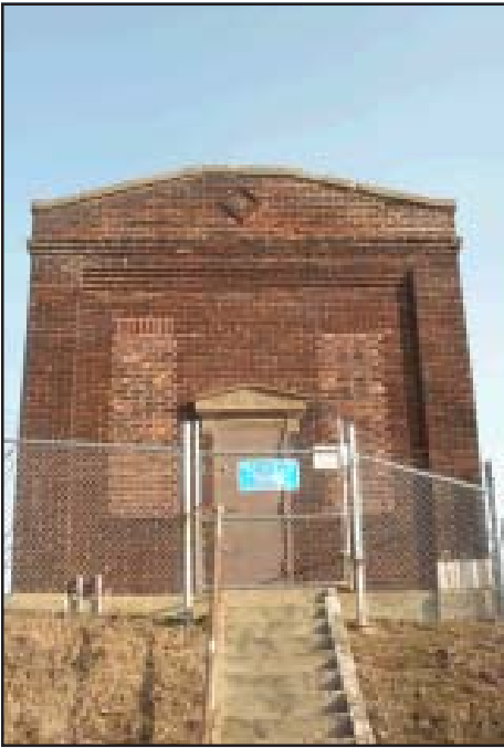
One of two gatehouses on the site, which will be demolished along with the reservoir.
