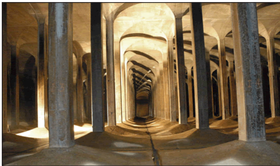
A reservoir in Roseville, part of the St. Paul Regional Water Services, is being demolished after more than 90 years of service. See page 3 for the full story.
