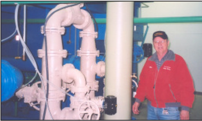
Mike Albrecht in the new La Crescent water treatment plant.
