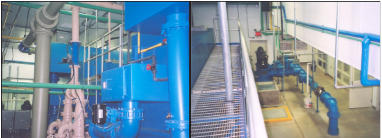
The two gravity filters and pipes in the new water treatment plant in La Crescent.
