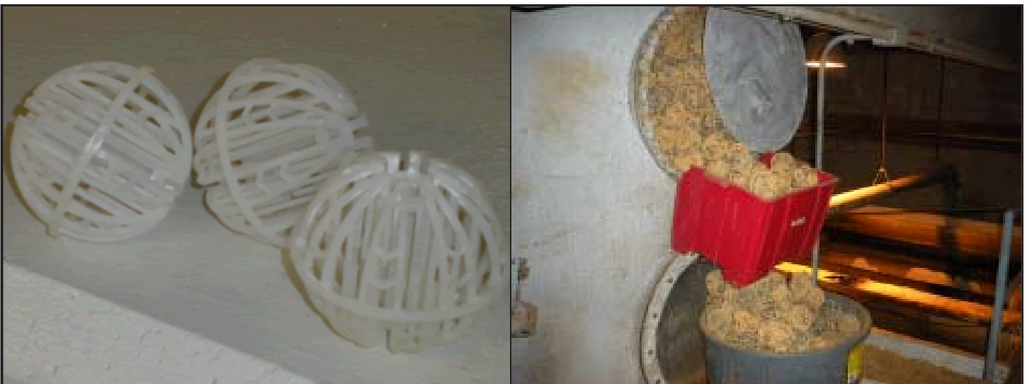
The air stripping towers are packed with hollow balls to remove contaminants. The photo at right shows fouled balls coming out of the air stripping tower in the original plant, which is no longer in service.
