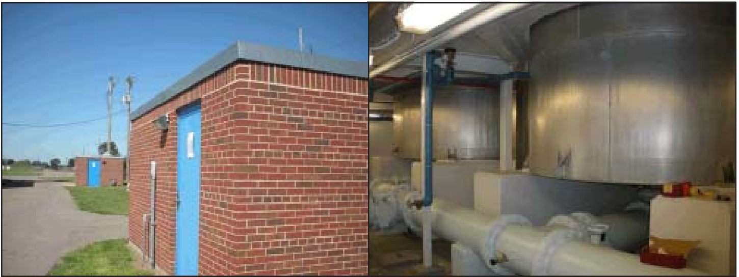
Wells 1 and 3 are in back of the old plant (left). Photo at right shows the base of the air strippers in the existing treatment plant.
