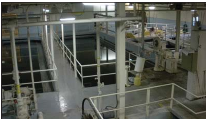
The filters at the existing Fairmont water treatment plant.
