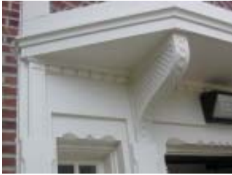
Decorative bracket of the 1927-28 Hall Pavilion bay window designed by architect Clarence H. Johnston
