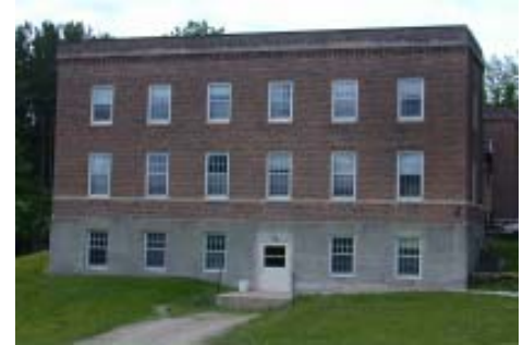
The basement level of Lakeside Pavilion is highly usable with its on-grade access and adequate windows providing natural light.
