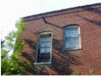
The old Pump House building near the lakeshore has distinctive features and location for creative new uses, but is vacant and deteriorating.
