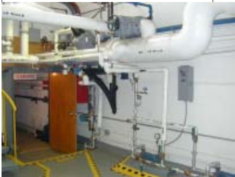
Underground tunnels (top) route utilities throughout the AGCC campus. The Power Plant (above and above right) provides service adequate for full occupancy of the programs, now utilized below capacity.
