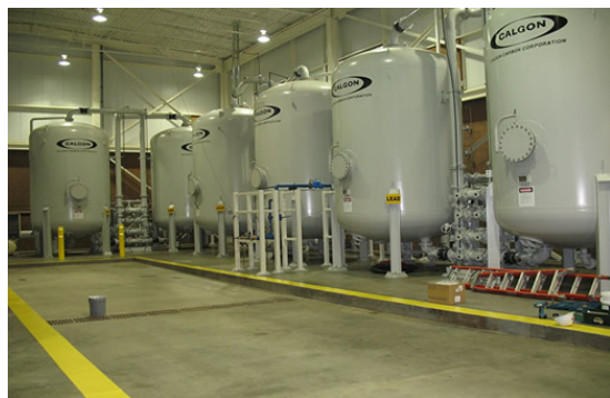
Image: City of Oakdale water treatment plant
