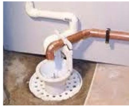
Drainage of the softener discharge line to a floor drain with an air gap
