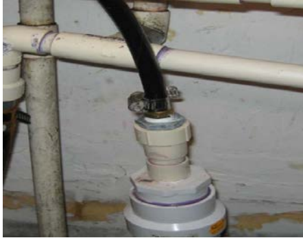
Softener discharge drain line directly plumbed to a sewer
