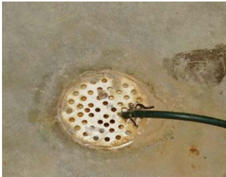
Drainage of the softener discharge line to a floor drain without an air gap
