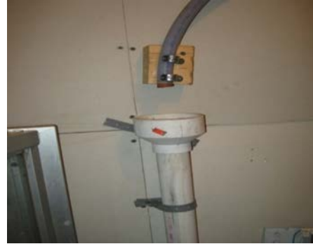
Softener discharge drain line with air gap
