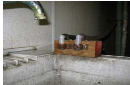
Placing the softener discharge drain line into a sink with an air gap
