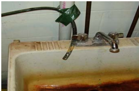
Placing the softener discharge drain line into a sink without an air gap
