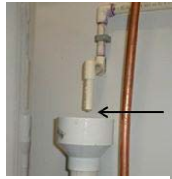
Air gap in softener backwash drain line
