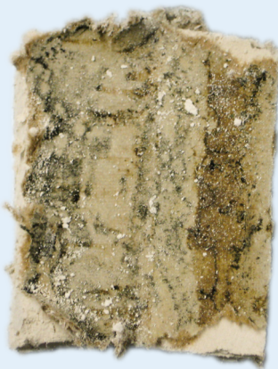
Mold growing on drywall. The drywall should be removed.
