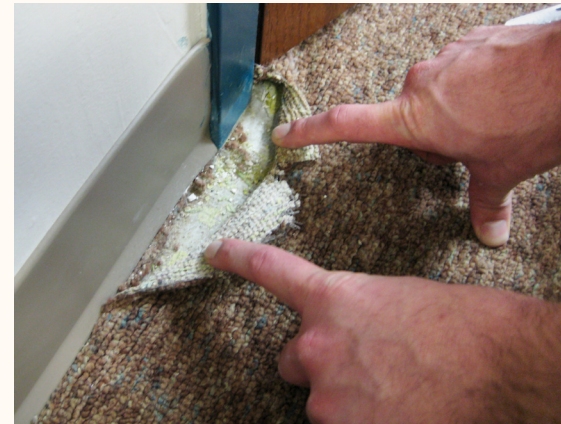
A thorough inspection, including peeling back carpeting, may find mold growth.
